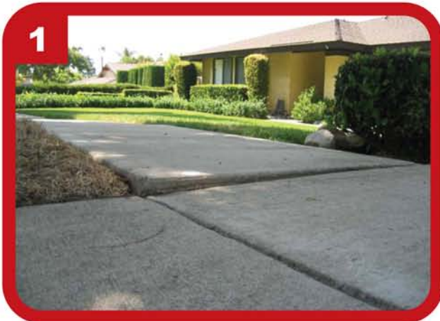
1 Survey to identify trip hazards
