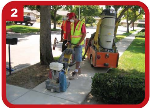
2 Grind trip hazards
